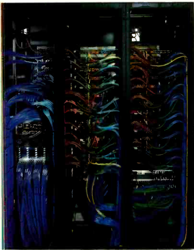
Rear view of routing rack.
